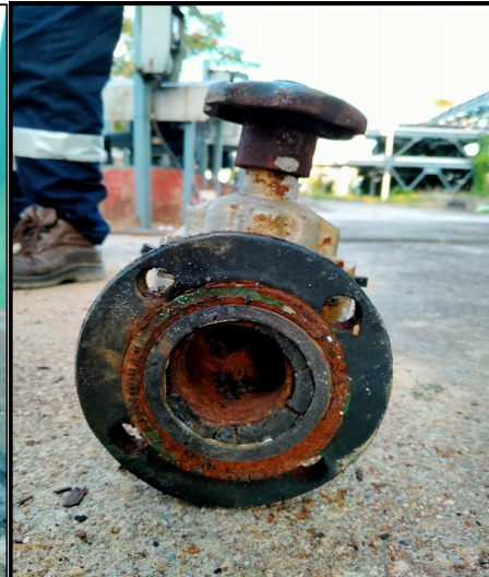
Figure 4: Pump recirculation iso valve
