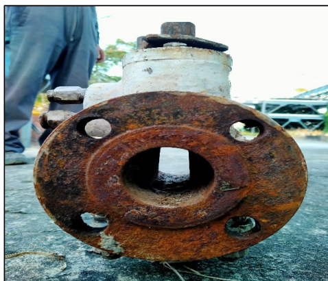
Figure 5: Pump suction root iso valve
