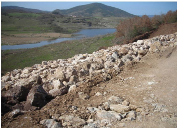
Figure 2: Protective Measure Against Flooding: Rip Rap on Embankment Slope
