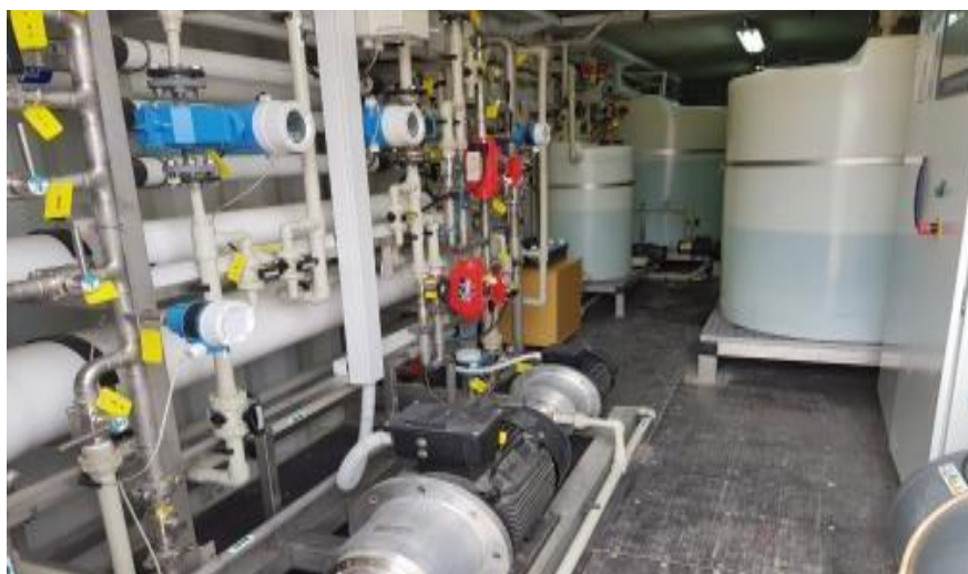
Figure 1: Pilot Plant on KACST 3 m 3 /d
