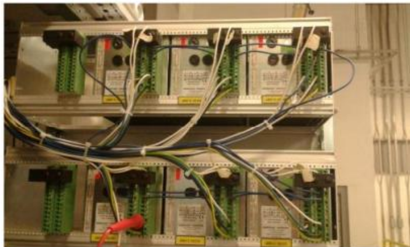
Figure 7: Rear Photo of LB 440 Evaluation Units Installed on the Panel
