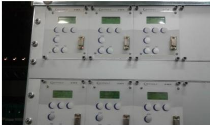
Figure 6: Front Photo of LB 440 Evaluation Units Installed on the Panel
