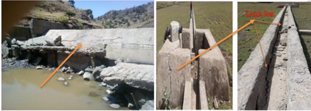
Figure 4.3. Terari Small Scale Irrigation Project Design Quality Problem
