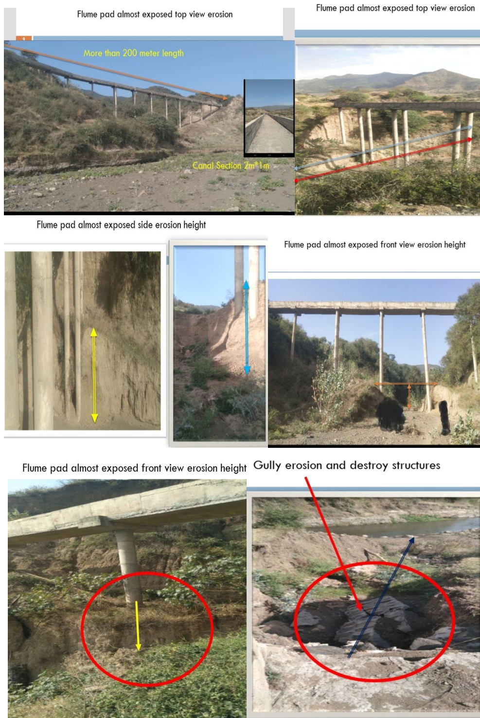
Figure 4.1. Mile Kotech Irrigation Project Flume & Gully Structure Quality Problem
