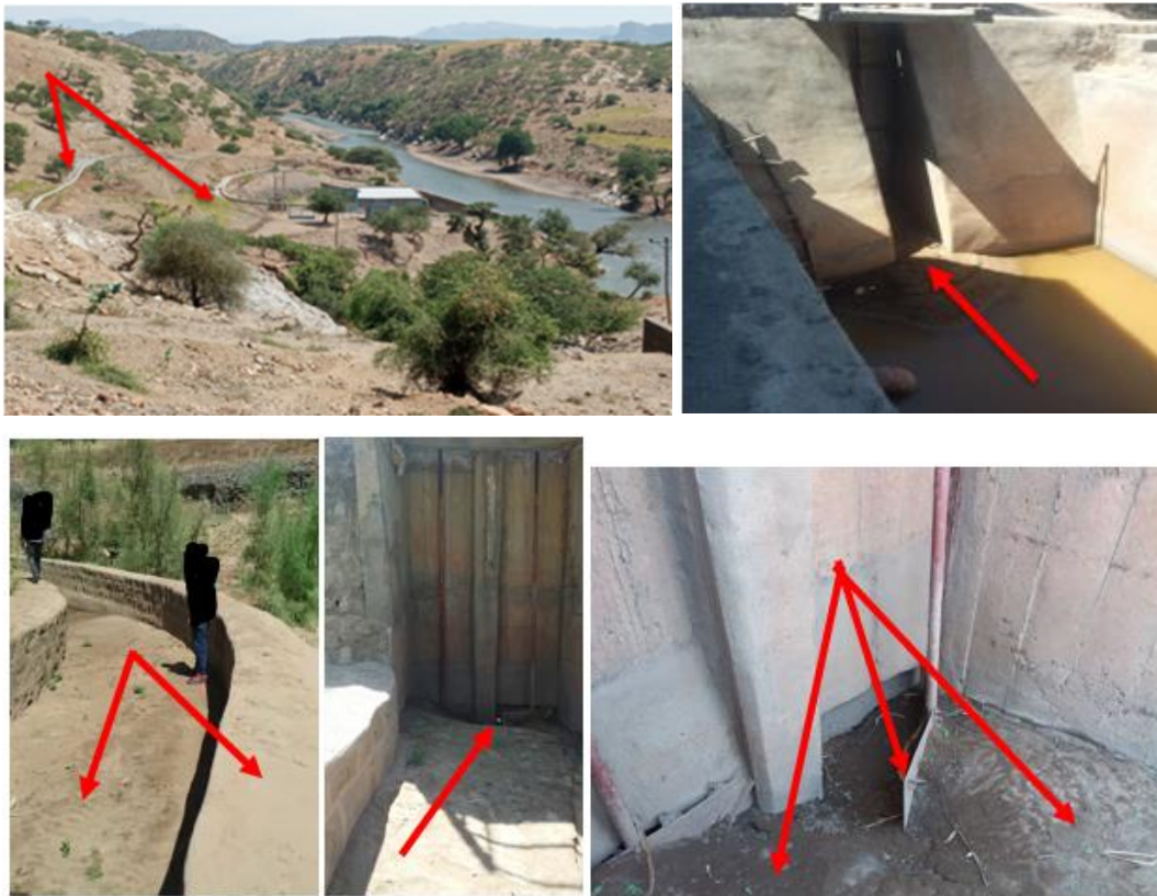
Figure 4.2. Zamra Small Scale Irrigation Project Design Quality Problem
