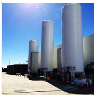
Figure 6: Big tanks of cryogenic oxygen
