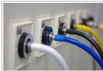
Figure 2: Medical gas pipeline system
