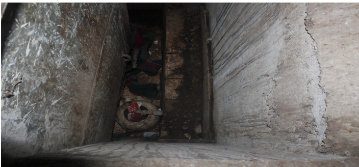
Blanket piece inside lavatory of the cell which were used as ligature material
