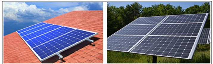
Figure 1: Roof Top mounted and Fixed Tilt Ground mounted PV Panels.
