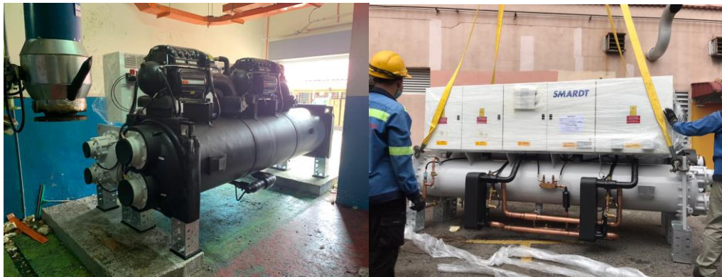
Figure 4: Oil-Free Compressor for Chiller System during Retrofit Program by Energy Performance Contracting with zero initial capital cost
