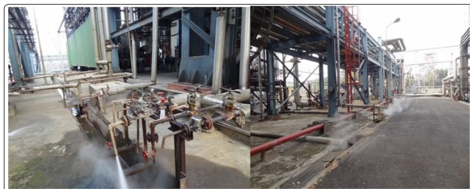
Picture 1: Area between UB & STG Pic-2: PRDS area
