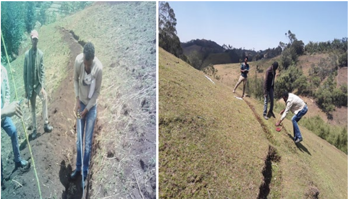
Figure 5: Field measurement on soil bund a) Hadiya b) Dawro Zones (Source; field survey)
