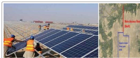
Figure 1: Pakistan solar power plant (Chinese company) 2015 100 MW [3]
